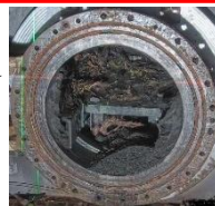
Status of deposits in the Unit 2 primary containment vessel (© Tokyo Electric Power Company Holdings, Inc.)
